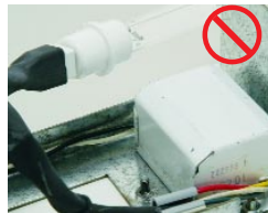
Many UV units use old fashioned ballasts that waste energy and have no monitoring
