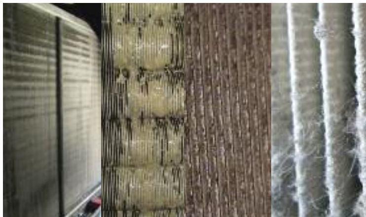
Bio-growth and mold coated coils accumulate debris and pass spores downstream to colonize on filters, ductwork and areas throughout the building.
